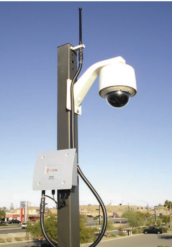
Security system at Yuma Airport
