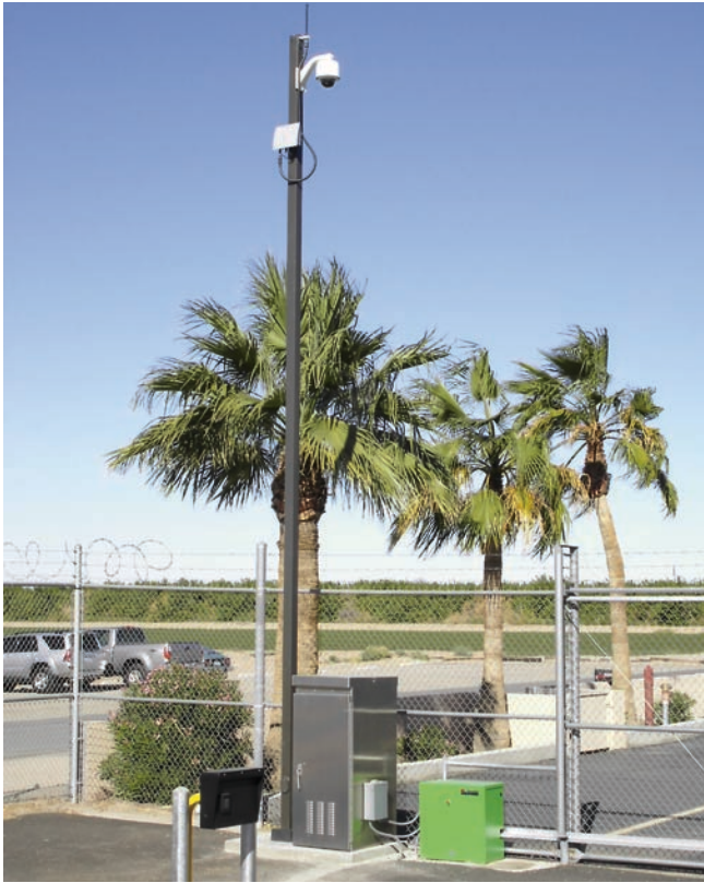
New access control and surveillance system powered by Firetide
